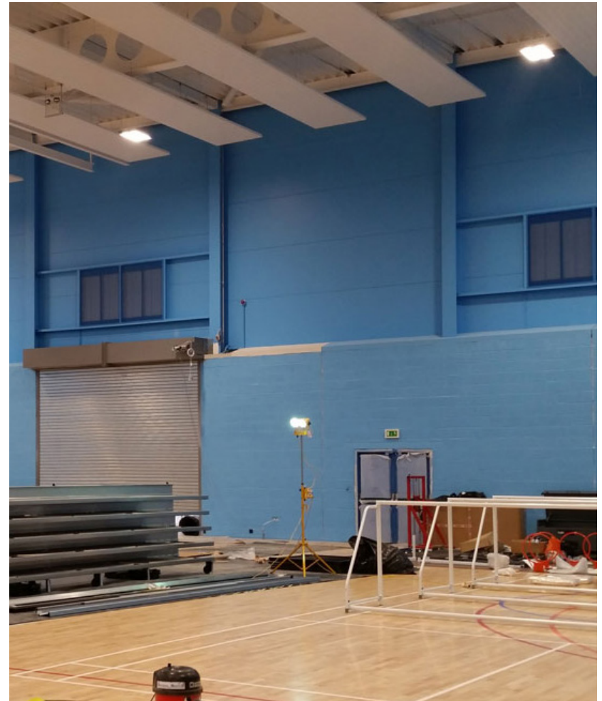
Windcatcher X-Air / Wycombe Sport Centre, High Wycombe
